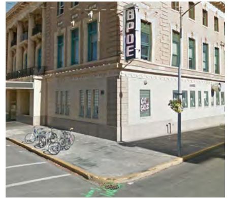
The northeast corner of the intersection of Front Street and Pattee Street lacks curb ramps for access from the street to the sidewalk
